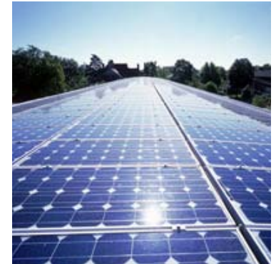
One of the world's largest solar-powered communities – Army Hawaii
